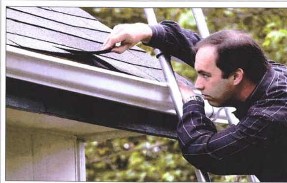
Home inspector Mark Panetti looks at the roof of a Burlington Township home. Panetti checks a house from top to bottom before it's sold. Photo by AL SCHILLI/Courier Post
